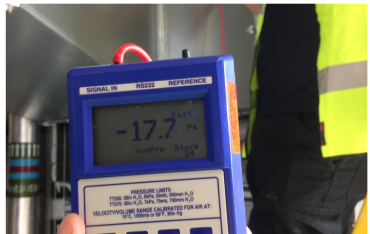
DOP HEPA Filter Integrity Testing
