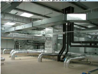
1st floor plant area with ductwork feeding Clean suite below and UPVC extract ducts from isolators
