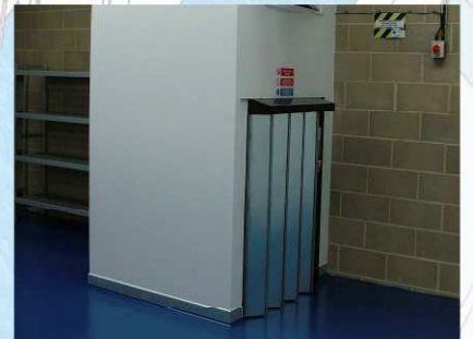
Goods lift to 1st floor store area
