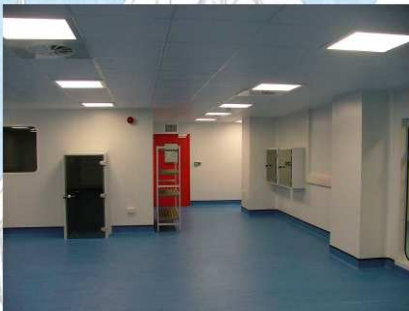
Grade D labelling and reconciliation cleanroom with trolley hatch and passthroughs
