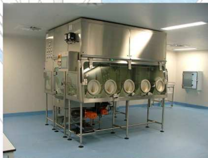
1 of 6 Twin isolators with rapid VHP unit Installed spread over 2 fully vinyl grade B rooms
