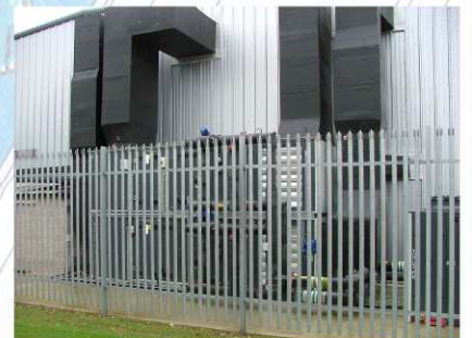
Exterior plant area with cleanroom and office air handling units
