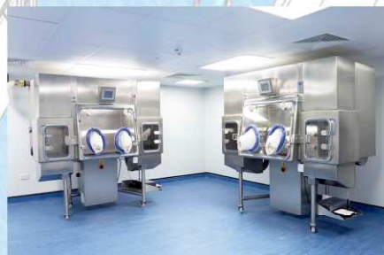
There are 2 isolators in each room 4 total and provision for a future isolator in each room
