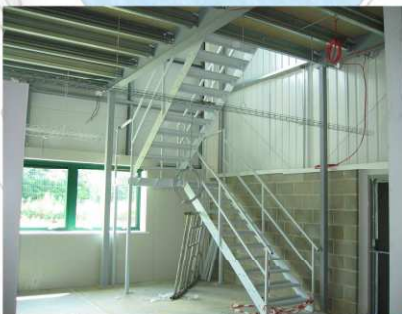
Installation of 316m 2 mezzanine floor including two fire escape stair cases and a goods lift
