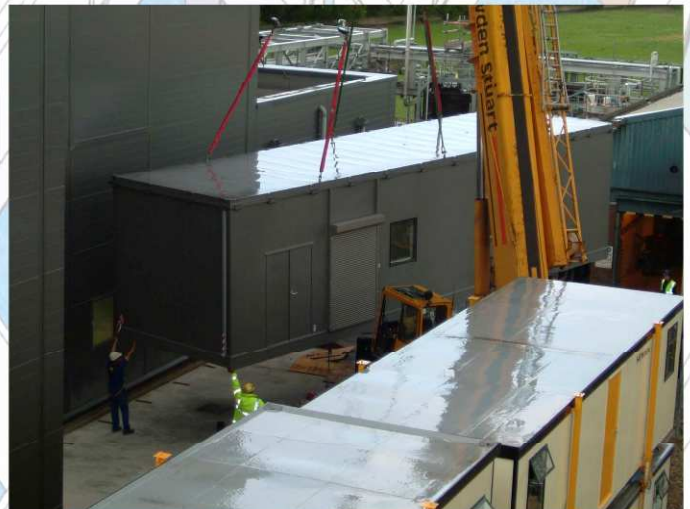
New modular building being craned into position finished to match existing building
